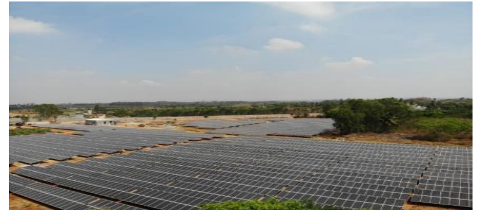
Solar Panels at HRGRDC, Bengaluru
