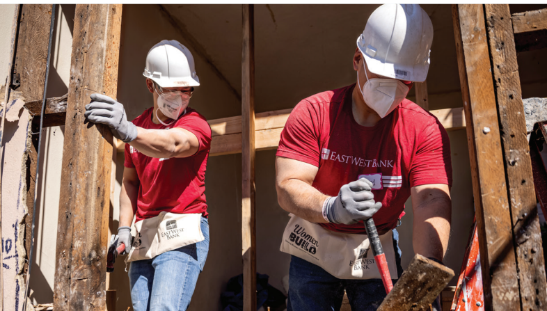
East West Bank partnered with San Gabriel Valley Habitat for Humanity to help build new homes for those affected by the Eaton Fire.
